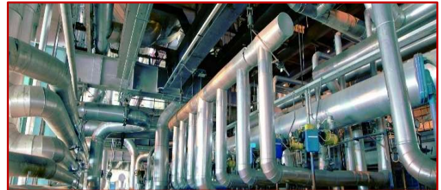
Piping, E quipment
